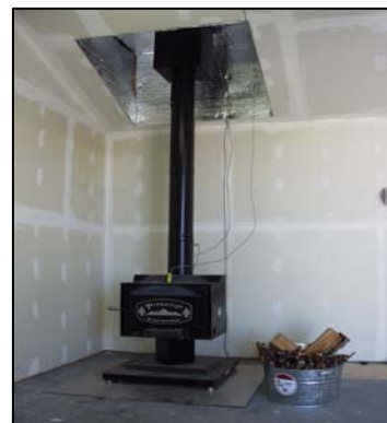
Figure 4. Wood stove and flue
